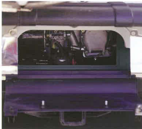
Rear licence plate generator access
