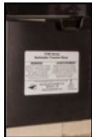
AUTOMATIC TRANSFER SWITCH
