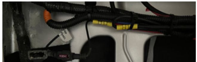
30 amp auto reset Breaker back of DCD
