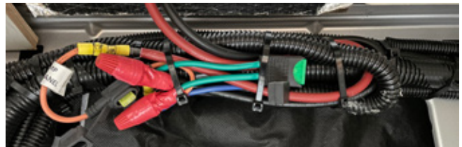
Fuse behind the microwave
