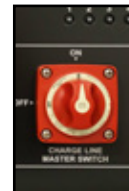
CHARGE LINE DISCONNECT
