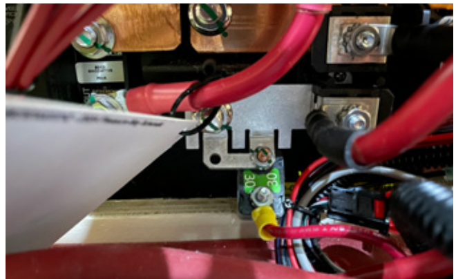
30 AMP AUTO RESET BREAKER BACK OF DCD
