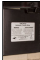
AUTOMATIC TRANSFER SWITCH
