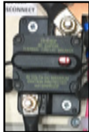
80 AMP CHARGER INPUT BREAKER
